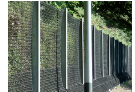
St. Georgen - St. Gallen (SG) Steinschlagnetze / Filets pare-pierres / Falling rocks nets
