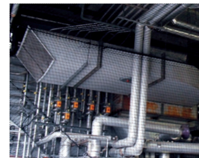
Novartis, Basel (BS) Anlagenschutznetze / Filets de protection des installations / Installation protection nets
